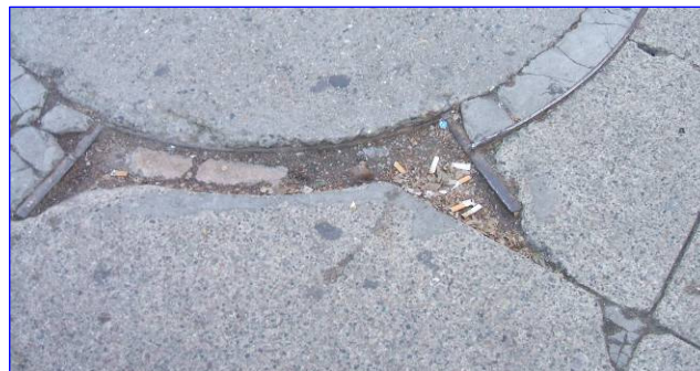
Figure 1. Cracked Sidewalk and cigarette butts by Park Street Station
