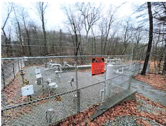
View of permanent gas easement
