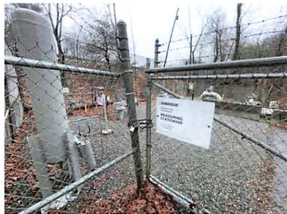
Alternate view of gas line infrastructure
